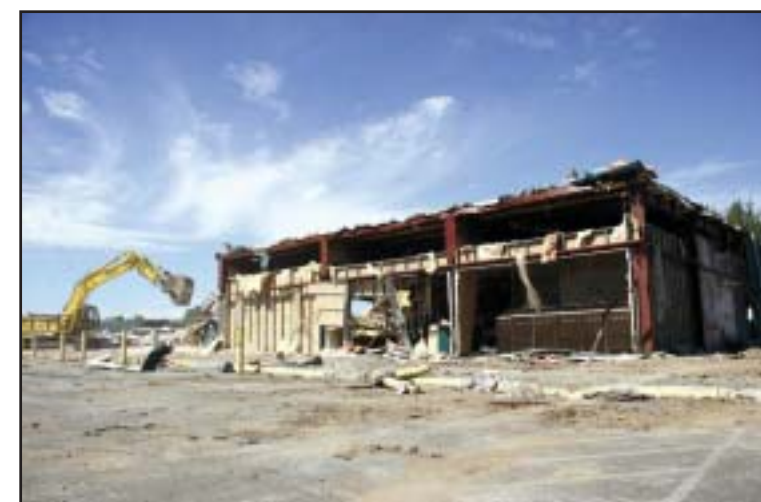
New beginnings - moving into the new facility means saying good-bye.
